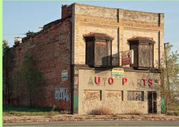
Figure 10.2 This dilapidated auto supply store in Detroit is a victim of auto industry outsourcing. (Photo courtesy of Bob Jagendorf/flickr)
